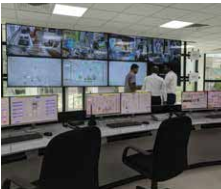
The Central Control Room at the Centre for Technical Excellence
