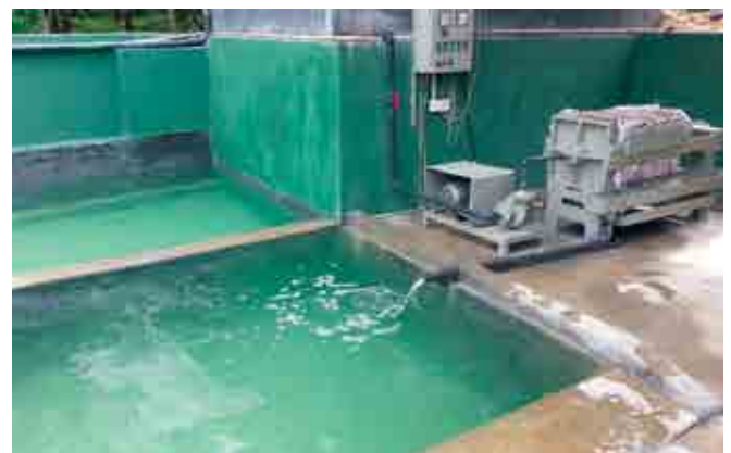
Storage tanks used for water recycling
