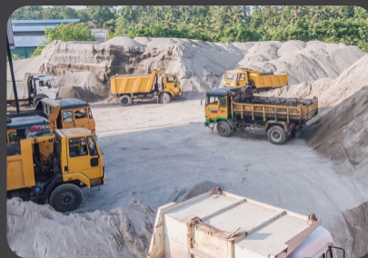
Commissions TOKYO SUPERSAND, a manufactured sand production plant that can produce 6000 Cubes of sand per month, with a crushing capacity of 100 MT/h.
